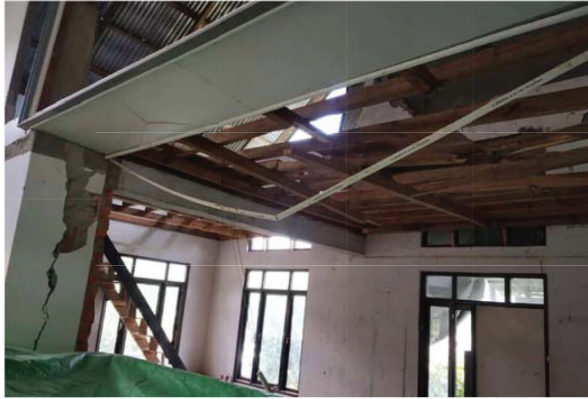
Fig. 3. Damaged community hall
