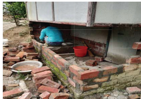
Fig. 2. Damaged sewer and pipe fittings
