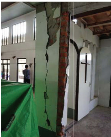
Fig. 5. Damaged residential house
