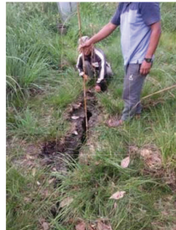
Fig. 6. Surficial cracks in Vaphai
